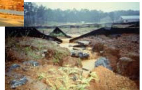
IMPROPER MAINTENANCE OF SILT FENCES CONTRIBUTES TO SOIL EROSION
