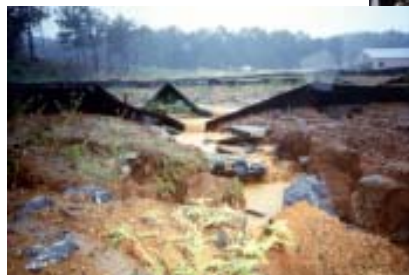
INADEQUATE BMPs CONTRIBUTE TO SOIL EROSION
