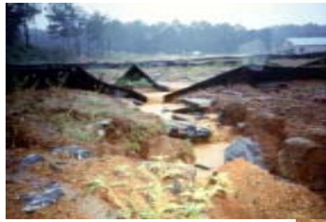
INADEQUATE BMPs CONTRIBUTE TO SOIL EROSION
