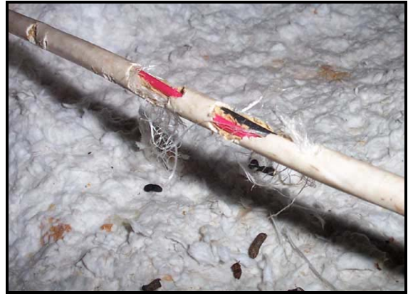
Rodent Gnawing Damage
