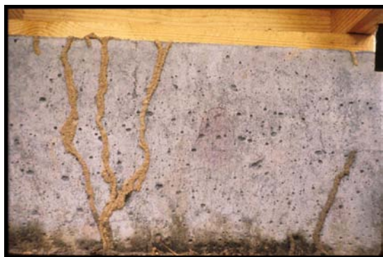
Termite Mud Tubes
