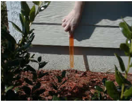
Fig. 1. An inspection gap between mulch and siding on the home will allow anyone to see if termites are building mud tubes into a structure.
