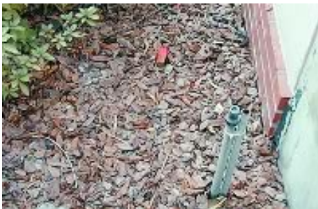
Fig. 2. Mulch that is too thick and obscures an inspection space will result in what is termed a “conductive condition” in the pest control industry. Irrigation heads that “water walls” is also considered a conducive condition.
