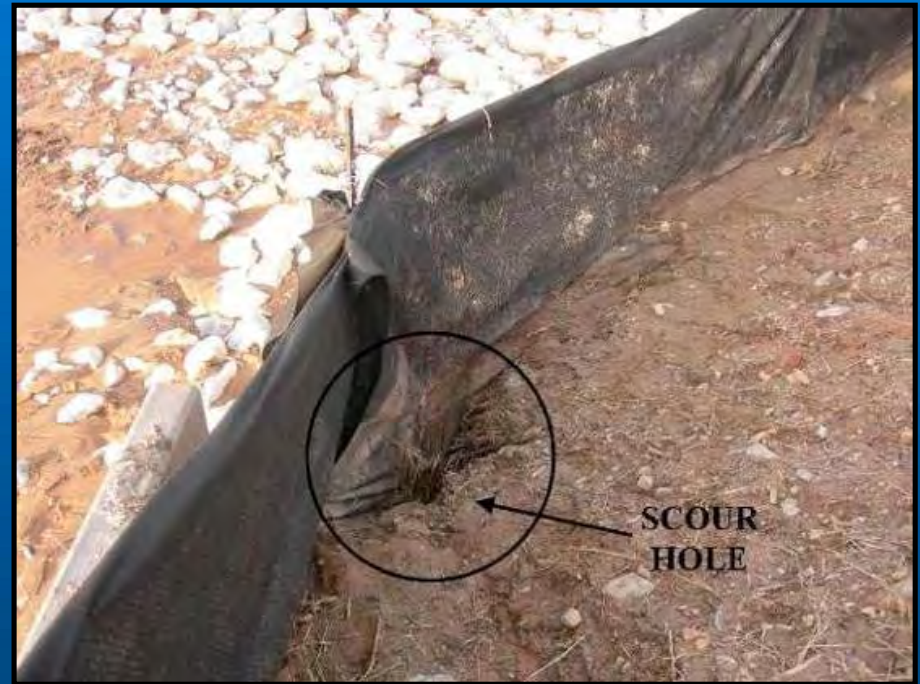
Downslope End: After (Scour Hole)
