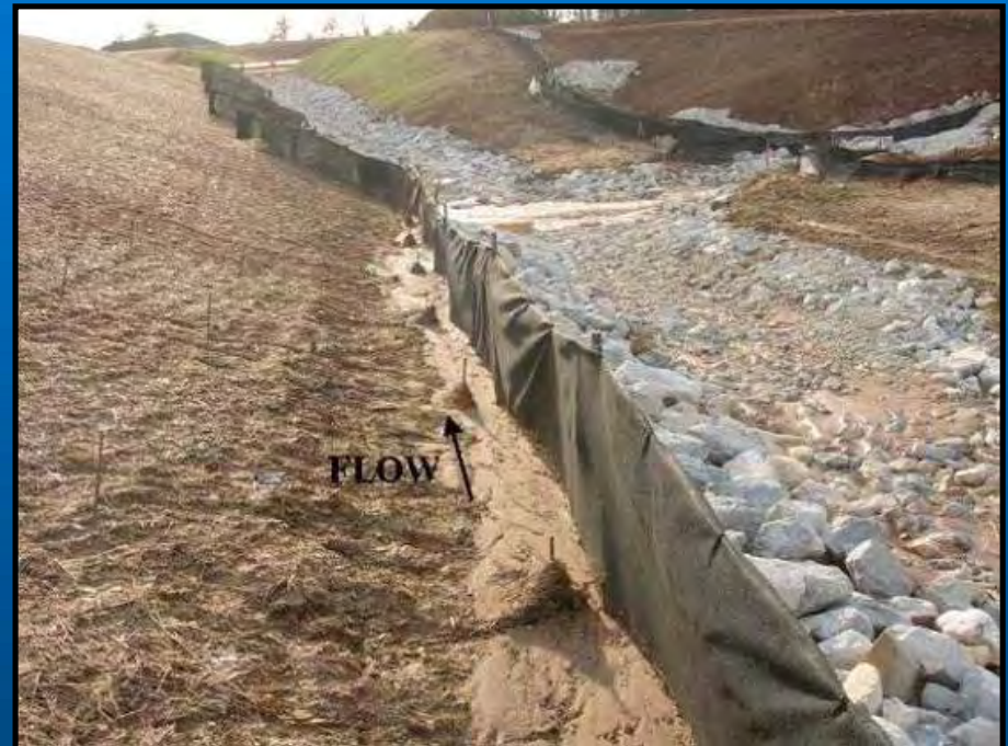
Downslope End: Heavy Sedimentation
