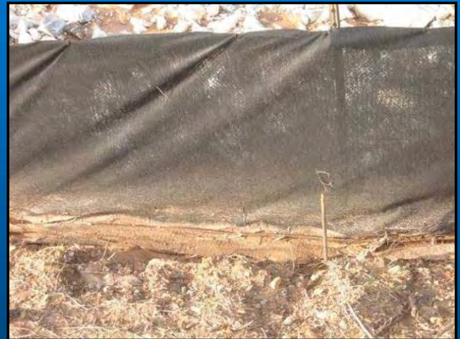
Erosion Along Toe of Fence
